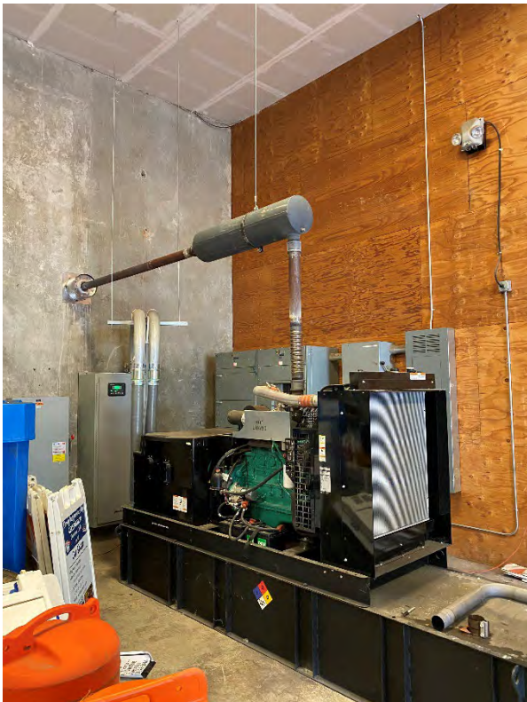
Ventilating the Public Works Warehouse Generator
